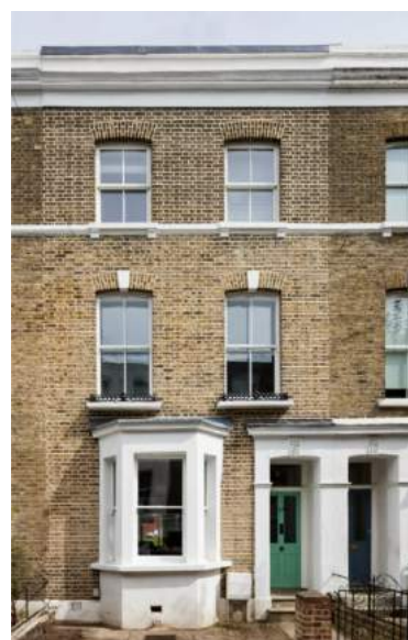
An example of a house fitted with various enhanced glazing. New double-glazed sashes on the second floor, secondary glazing to the first and new double glazing into old frames on the ground.
